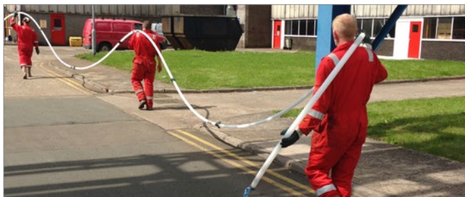
Nineteen 7-Channel CMT Systems were installed inside a manufacturing facility to characterize and monitor a plume beneath the building that is migrating off site. Systems were installed using sonic drilling to 30 m (100 ft) depths. Challenging geology made drilling and installation tricky, however, all Systems were installed in two weeks.
