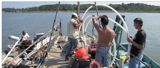
CMT Systems were installed at the bottom of a bay to measure submarine groundwater discharge. Eight 7-Channel CMT Systems were installed, with custom modifications to suit the open water application. Watertight wellheads had to be custom built to allow for sampling from the surface of the bay using a peristaltic pump.
